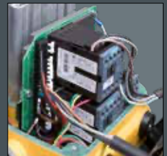
LOW VOLTAGE CONTROL
